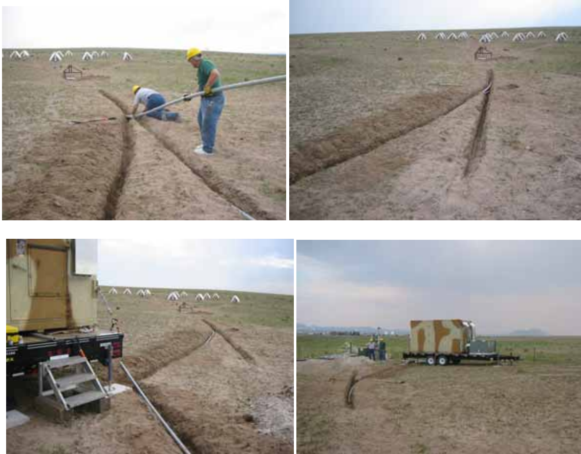
Figure 6. Photos showing the relocation of the two 2" conduit lines from the collector box at the array edge to fit the actual shelter location.
