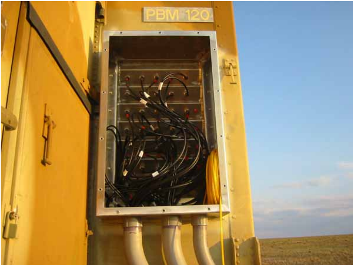
Figure 9. Photos of the incoming antenna cables at the shelter. Fiber is the yellow cable on the right of the bottom photo.
