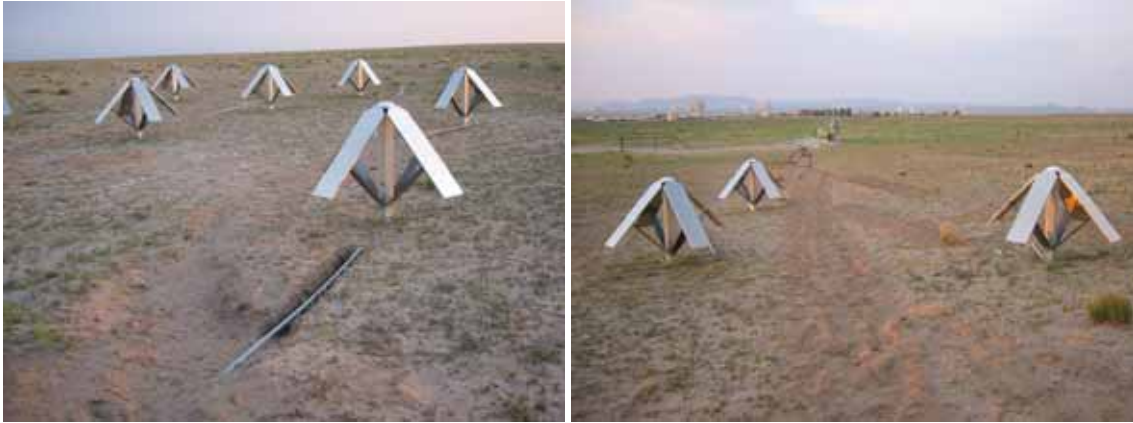
Figure 2. Photos showing the array and conduit runs that were previously installed.
