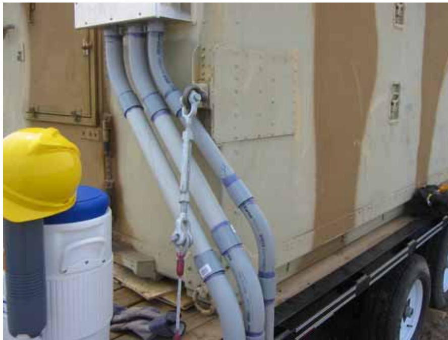
Figure 7. Top photo shows completed antenna and fiber conduit running to shelter patch panel. Bottom photo shows detail of the conduit meeting the patch panel, as well as one of the shelter tie-downs.
