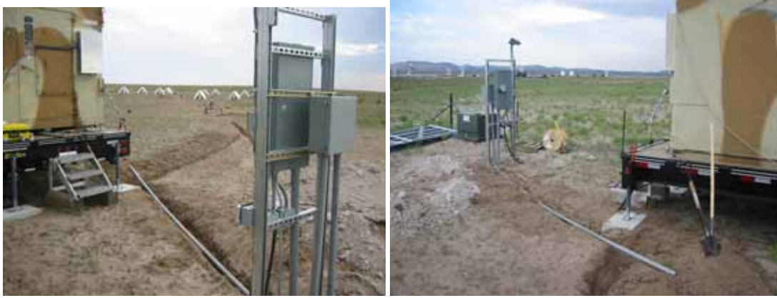
Figure 5. Photos showing the installation of the fiber conduit from junction box to shelter.
