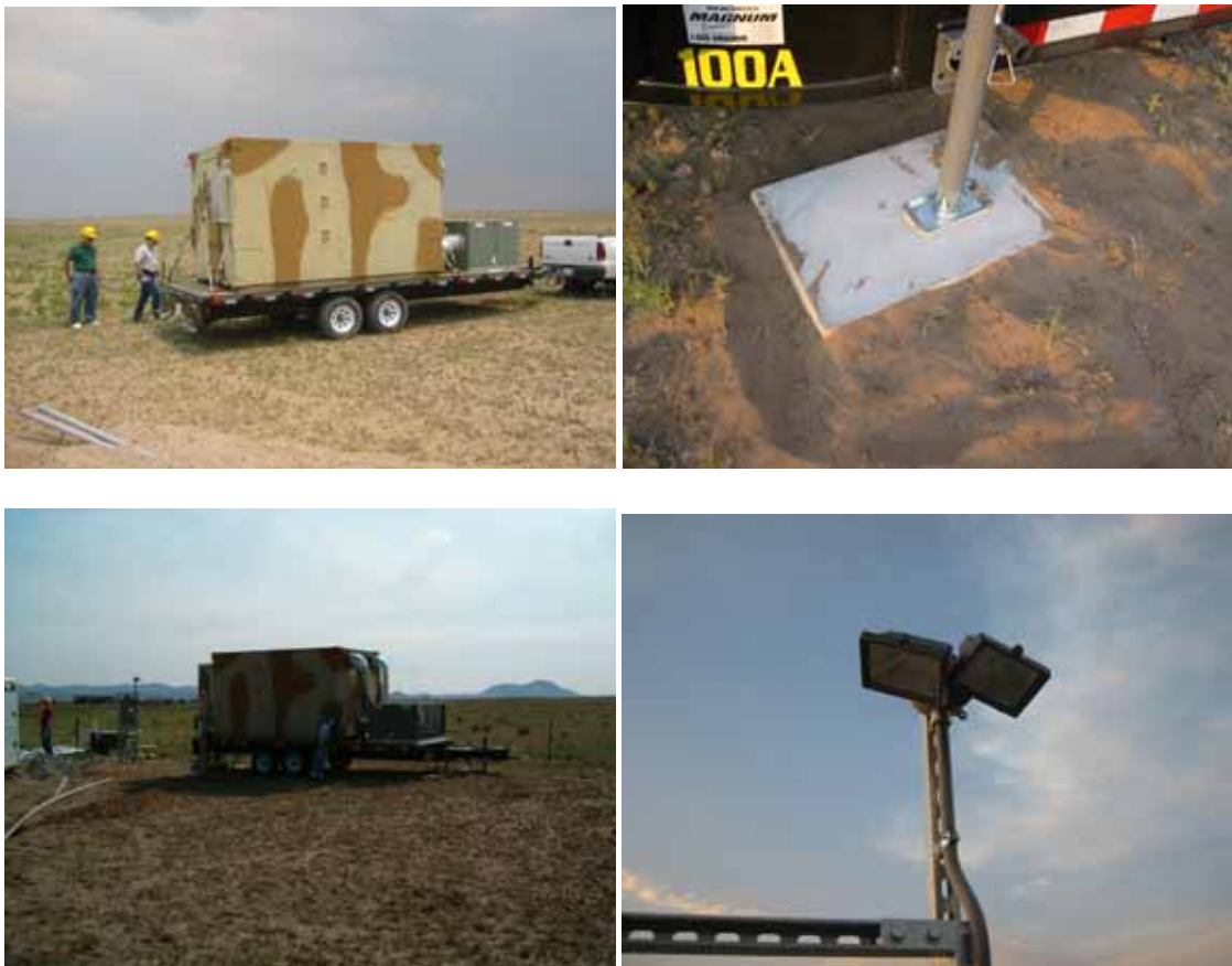
Figure 4. Photos of the shelter installation. Clockwise from top: positioning the shelter, concrete pad for the shelter jacks, the lights illuminating front of the shelter, and the final shelter location with the junction box at right.
