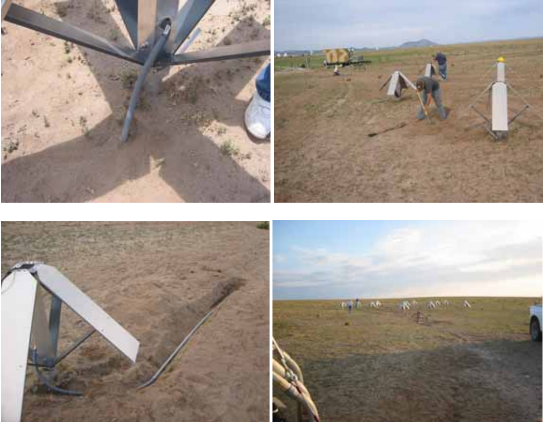
Figure 8. Clockwise from top left: 1) flexible conduit attached to antenna mast, 2) trenching for the final connection to the antennas, 3) looking out from the shelter to the completed (but filled) runs, and 4) a completed, unburied section, of the flexible conduit running to an antenna
